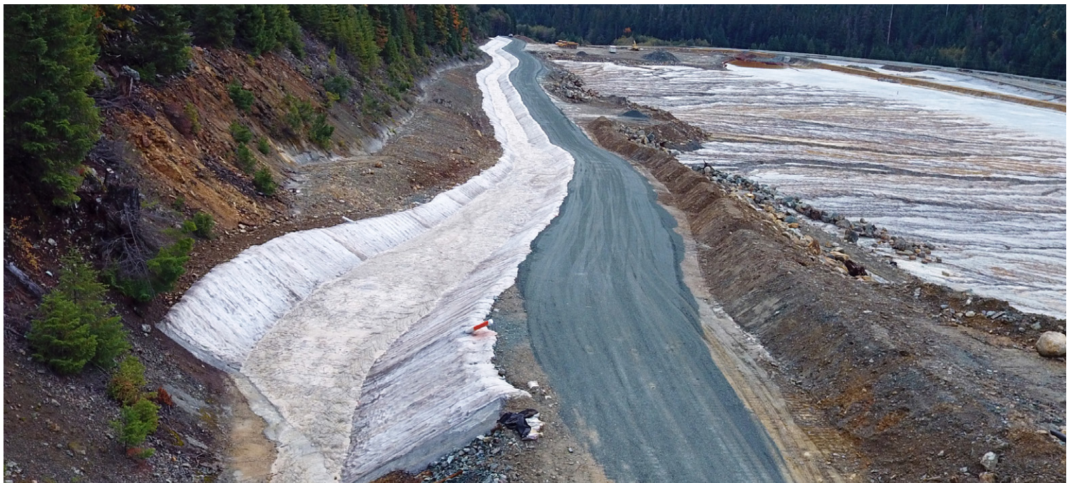
Aerial view of the mouth of the channel showing transition anchor trench
