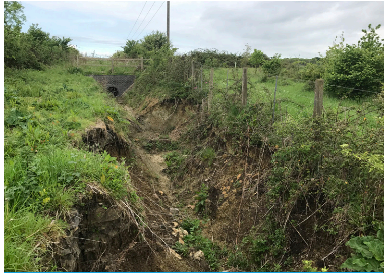
Unlined channel showing 3m deep scour and erosion
