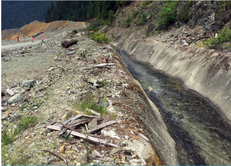
Previous shotcrete lined channel showing signs of degradation
