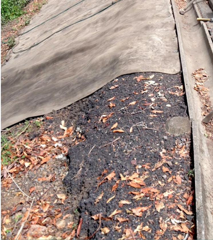
The existing slope liner had suffered erosion and damage
