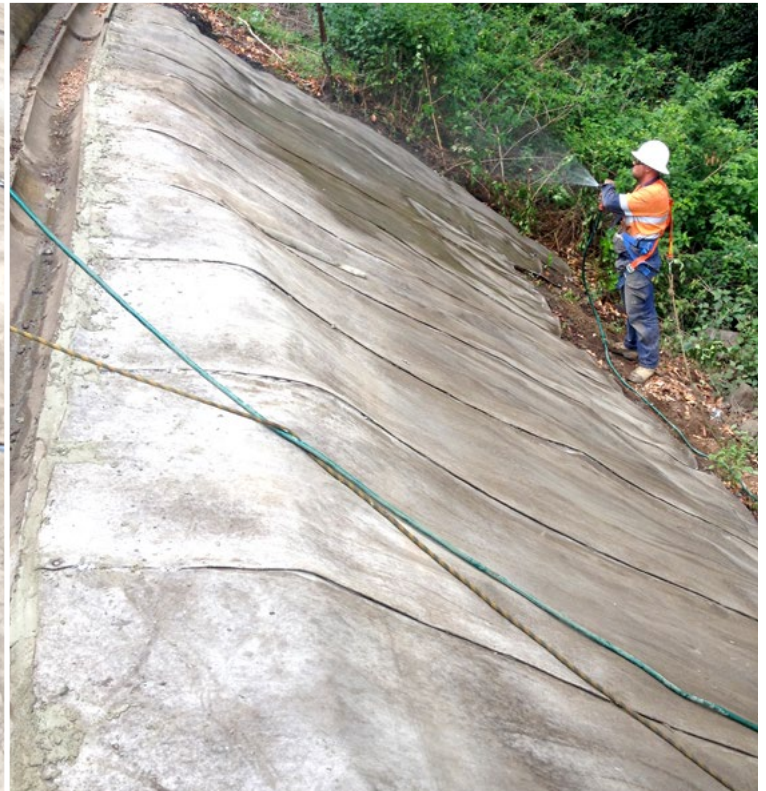
Grout was applied to the head of the slope prior to hydration
