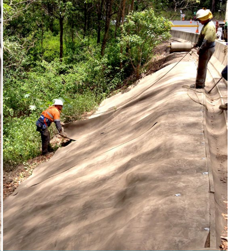
Bulk rolls of CC5 were dispensed using a spreader beam and crane truck
