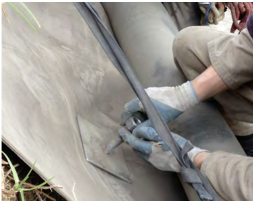
200x200mm steel plates were used to secure the CC to the slope face using the soil anchors.
