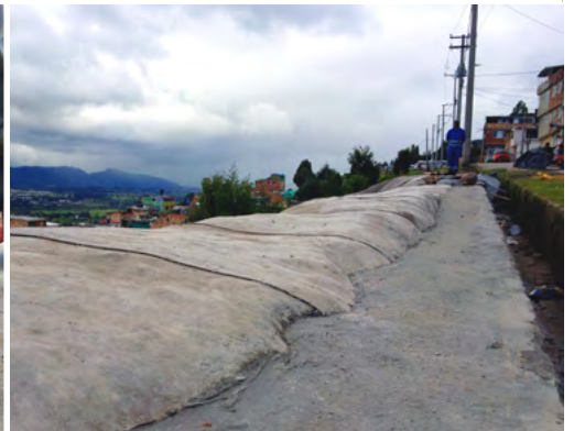
CC was secured at the crest with a concrete filled anchor trench.
