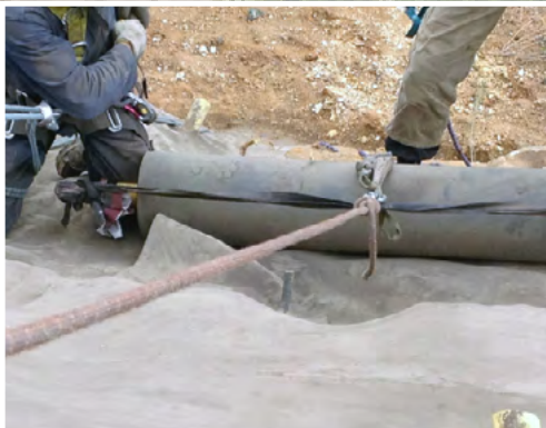
CC was dispensed from a spreader beam, allowing it to be laid at a rate of over 150m/day
