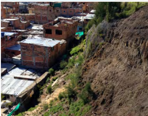
The project site before CC installation, showing severe erosion.
