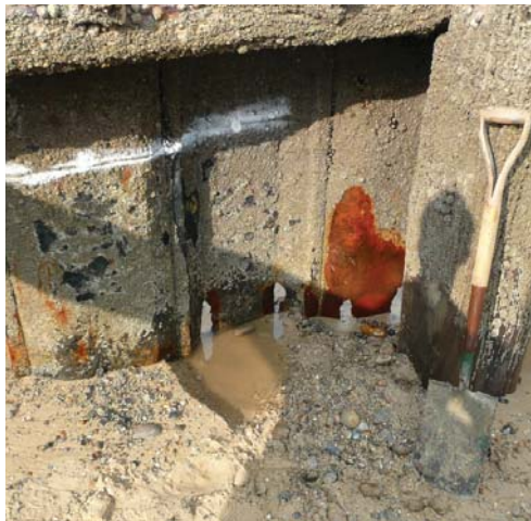
Groyne section in disrepair with dangerous voids
