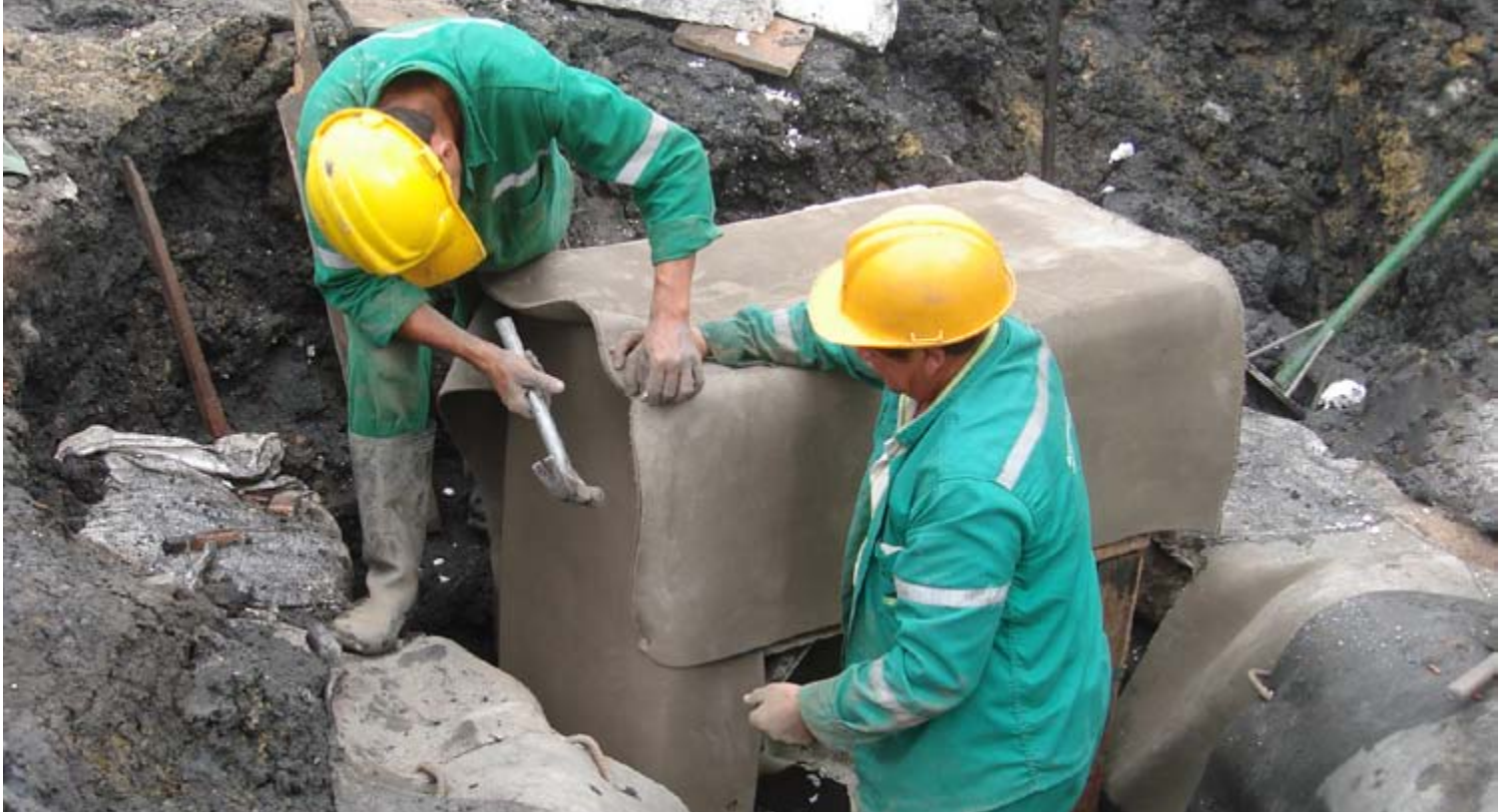
Lining a timber framework with CC to form a headwall at the top of the dissipater drain
