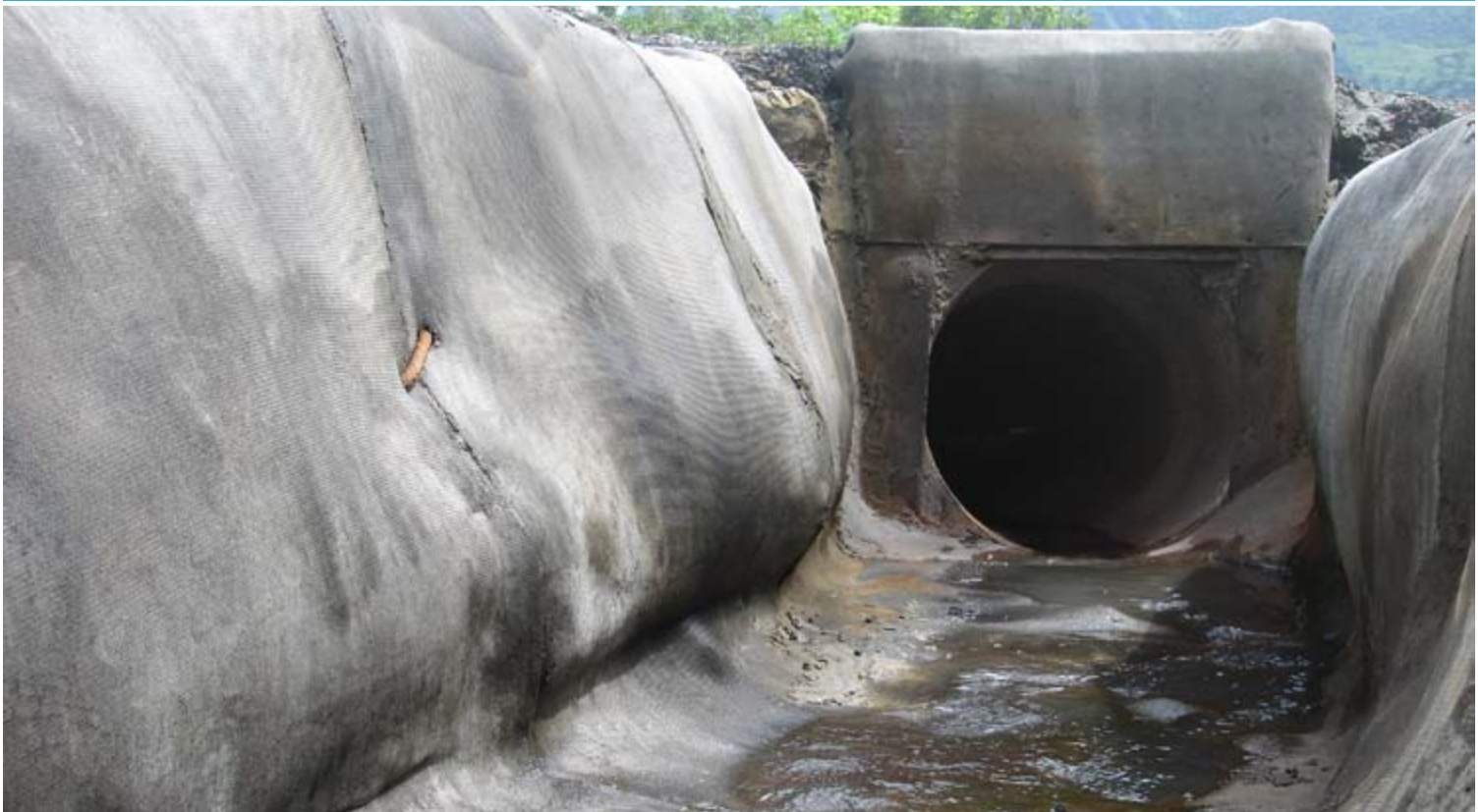
Photo of the lined drain section at the top of the dissipater drain showing how the CC conformed to the natural contours of the profile.
