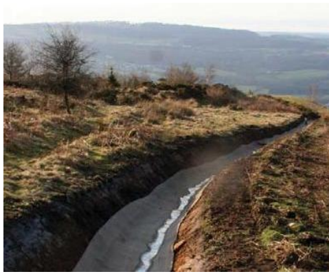
Ditch lining at Bedwas: Courtesy of Caerphilly Council
