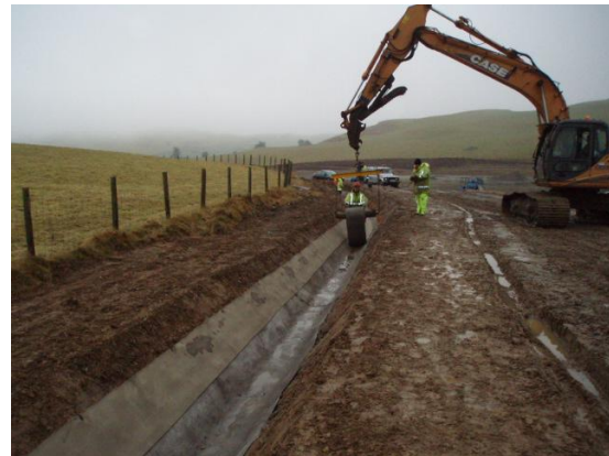
Concrete Canvas being applied to a channel: Courtesy of the Environment Agency
